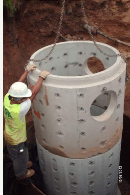
Leaching Catch Basins
